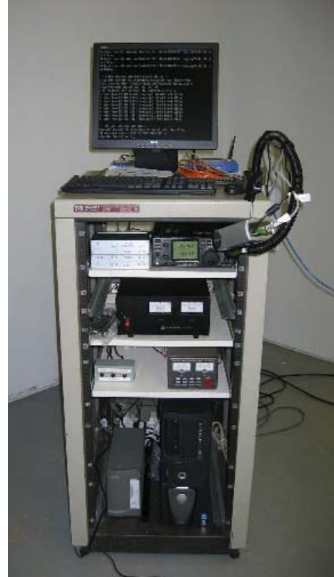
Ground Station Equipment Rack at Fairbanks
